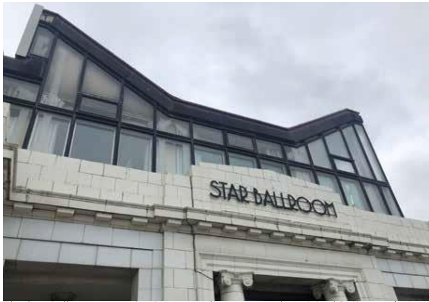
The Star Ballroom extension is uncomplimentary to the original Ballroom design. The heavy form sits awkwardly on top of the original building and dominates the beachfront façade.
